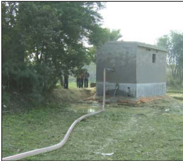
Pump House with Flexible Pipe for Irrigation Water
